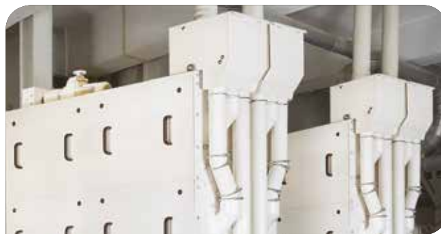
Line of two Rotosort™ in a large capacity rice mill - a modular DRGA-3D configuration
